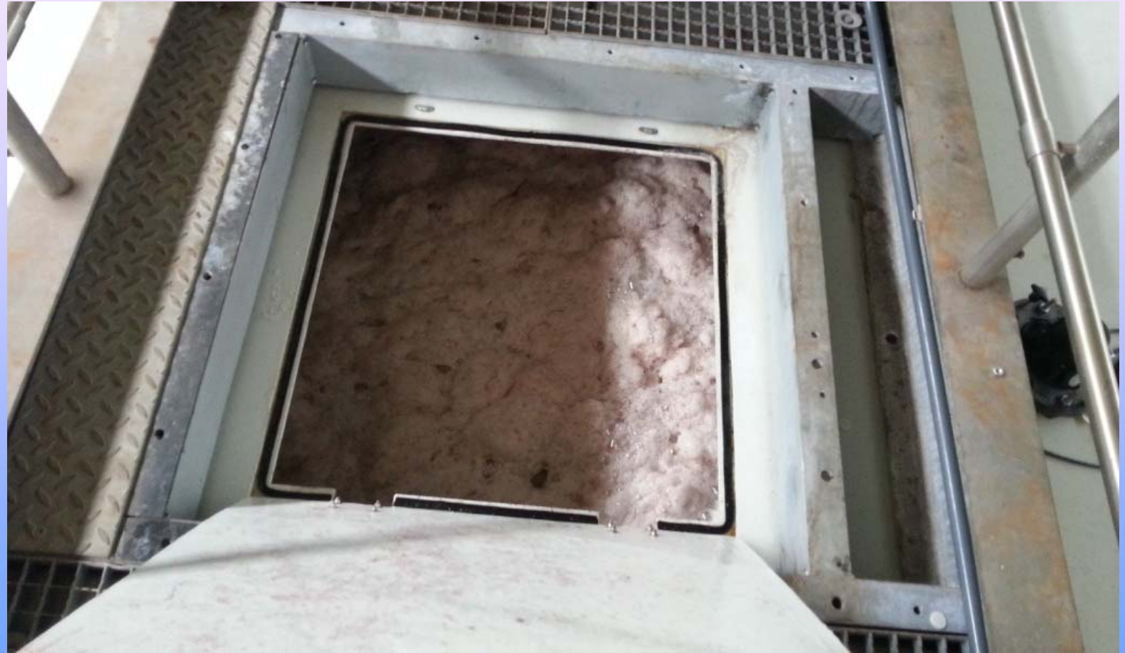
View into the Mutag BioChip™ MBBR tank
